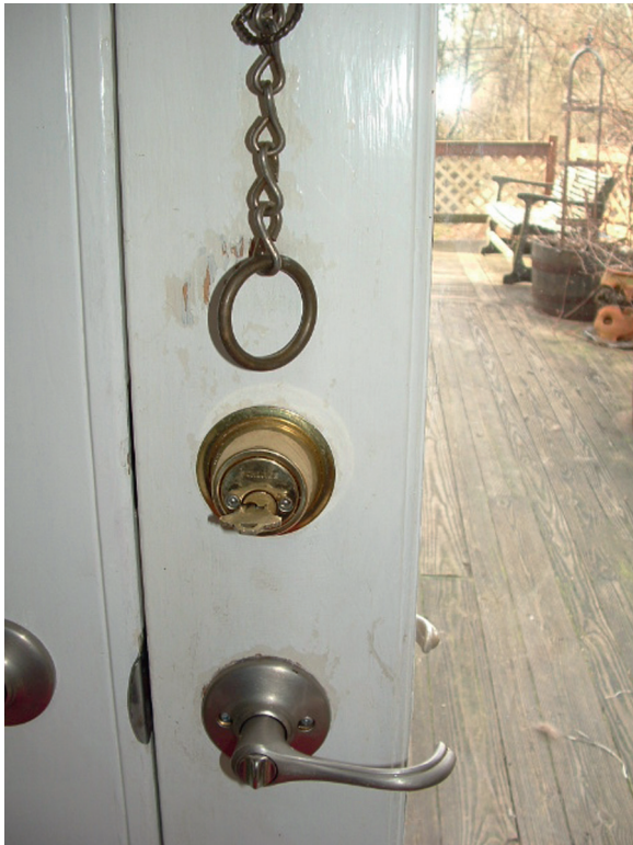
Some of the first signs of damage associated with separation anxiety may be seen on doors.
